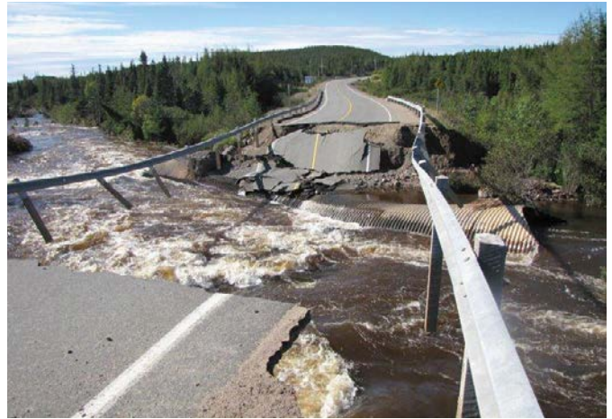
FIGURE 7: Damage to the highway and bridge near Port Rexton, NL due to Hurricane Igor. Photo courtesy of Fire and Emergency Services, Newfoundland and Labrador.
