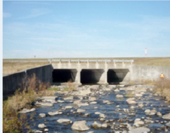
Figure 7: Spring Creek Triple Box Culvert at Pearson Airport. (Source: Toronto Pearson - Spring Creek Culvert, 2010 - Photo taken by Morrison Hershfield Limited and provided courtesy of the Greater Toronto Airport Authority)
