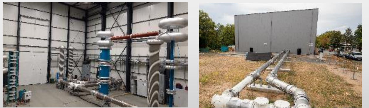
Figure 9: Test setup for long-term verification of the DC GIL in Darmstadt (left: voltage and current supply; right: electrical test setup); copyright Siemens AG, see also Hallas et al. (2020) 38
