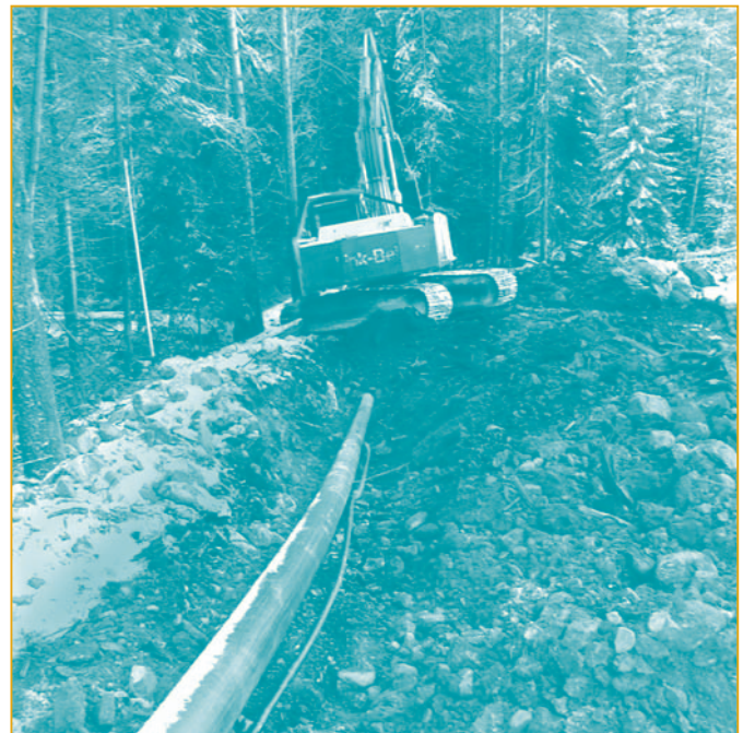
Figure 29. Burying a 20-cm (8-in.) Penstock pipe (photo courtesy of Thomson and Howe Energy Systems Inc.)
