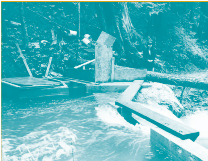
Figure 11. An intake weir for a 7-kW system (photo courtesy of Thompson and Howe Energy Systems Inc.)
