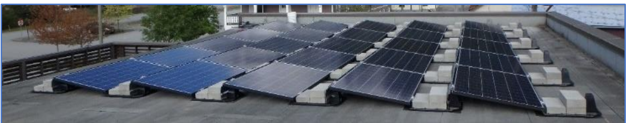
Figure 25: Example of a Flat Roof Ballasted Solar PV Array - courtesy Riverside Energy Systems
