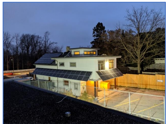
Figure 15: Residential Wall-mounted Solar PV system - courtesy of Blue Water Energy
