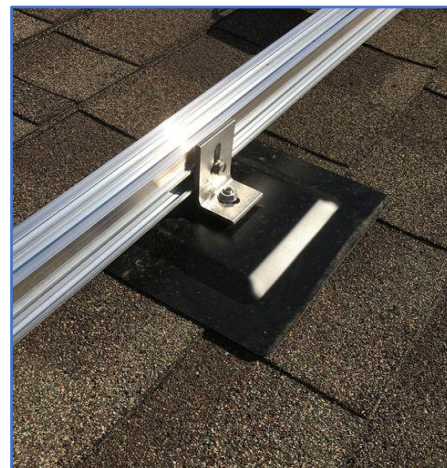
Figure 23: Flashed Anchors screwed to Roof Decking, with racking attached - courtesy Riverside Energy Systems
