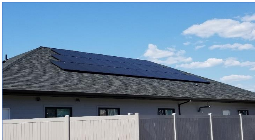
Figure 20: Intended 15 kWp System Limited to 10 kWp by Electric Service Panel Choice - courtesy of Riverside Energy Systems
