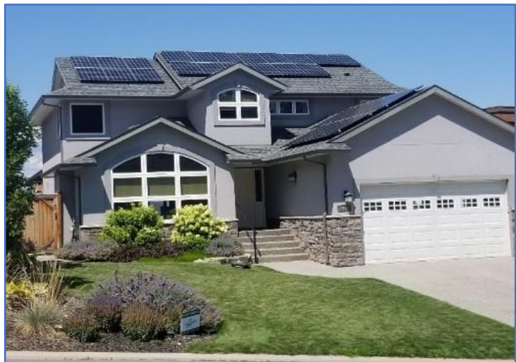
Figure 12: Roof Mounted PV System using South and West Facing Arrays - courtesy Riverside Energy Systems
