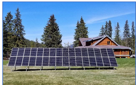
Figure 16: Ground-mounted Solar PV Array - courtesy of Riverside Energy Systems
