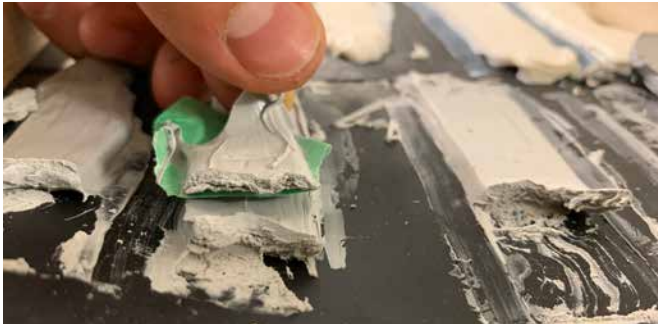
Figure 4 Example of cohesive failure of the sealant bead.
