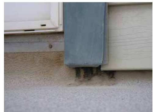
Figure 2 Signs of plasticizer migration from a self-adhered membrane through to the urethane-based liquid-applied membrane.
