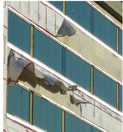
Figure 1 Damage to a non-adhered sheathing membrane during construction due to wind.
