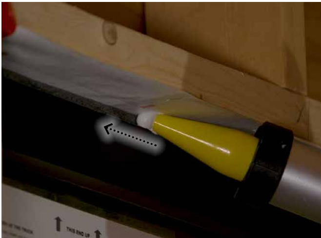
Figure 6 Example of correct installation and simultaneous tooling of sealant at window perimeter interface.
