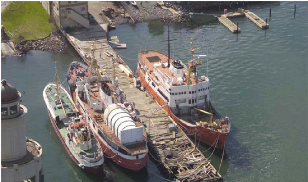
Figure 6: Storm surge causes wharf damage in Halifax Harbour. (Source: Environment and Climate Change Canada)
