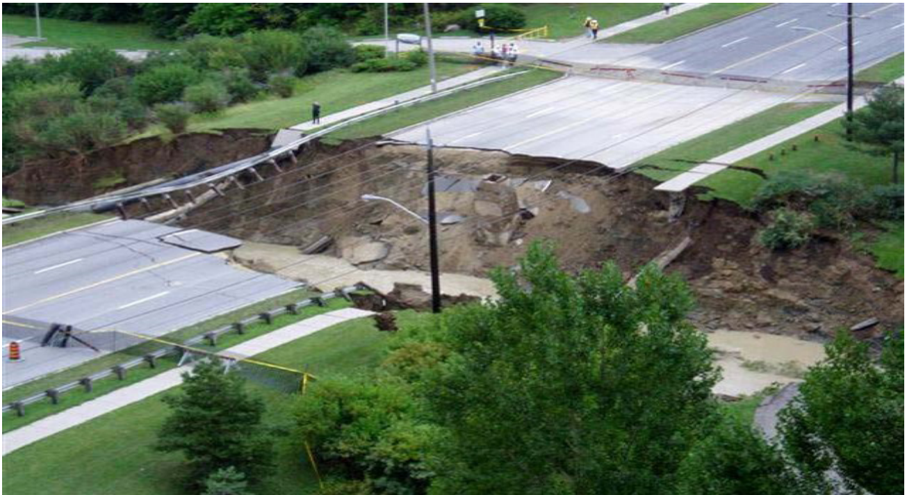
Figure 7: A section of Finch Avenue washed out during the heavy rainstorm of August 19, 2005. (Source: City of Toronto)
