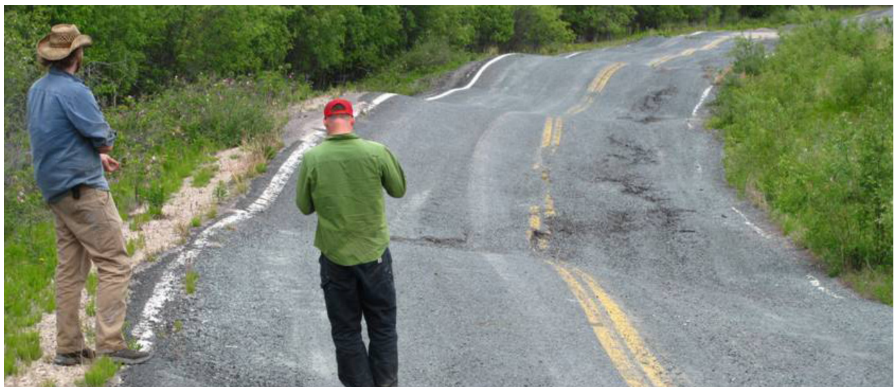
Figure 7: Differential settlement associated with permafrost thaw along an abandoned section of Northwest Territories Highway 4, east of Yellowknife. (Source: Natural Resources Canada)
