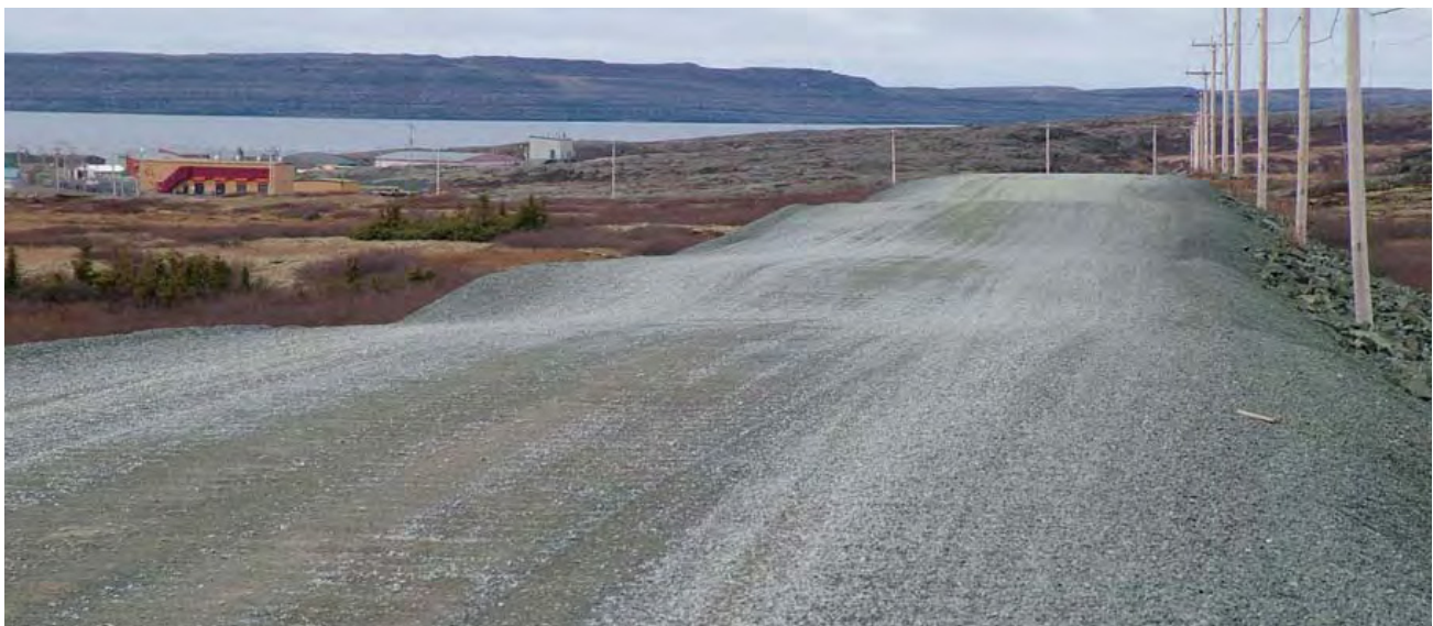
Figure 10: Significant settling on the Umiujaq access road. (Source : Allard, M., Fortier, R., Sarrazin, D. et al., 2007)
