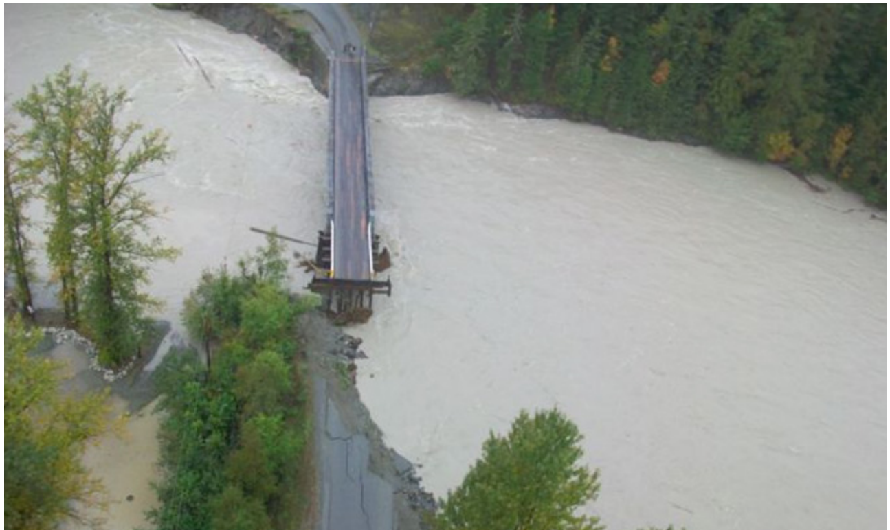
Figure 8: Bella Coola: Highway 20 Flood Impacts – Sallompt Road bridge approach washout. (Source: British Columbia Ministry of Transportation and Infrastructure)
