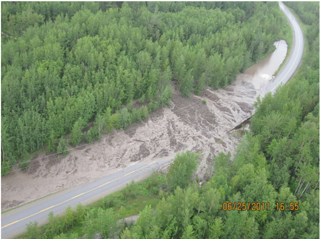
Figure 9: Pine Pass: Highway 97 Flood Impacts – Blocked road access between Pine Pass and Chetwynd. (Source: British Columbia Ministry of Transportation and Infrastructure)
