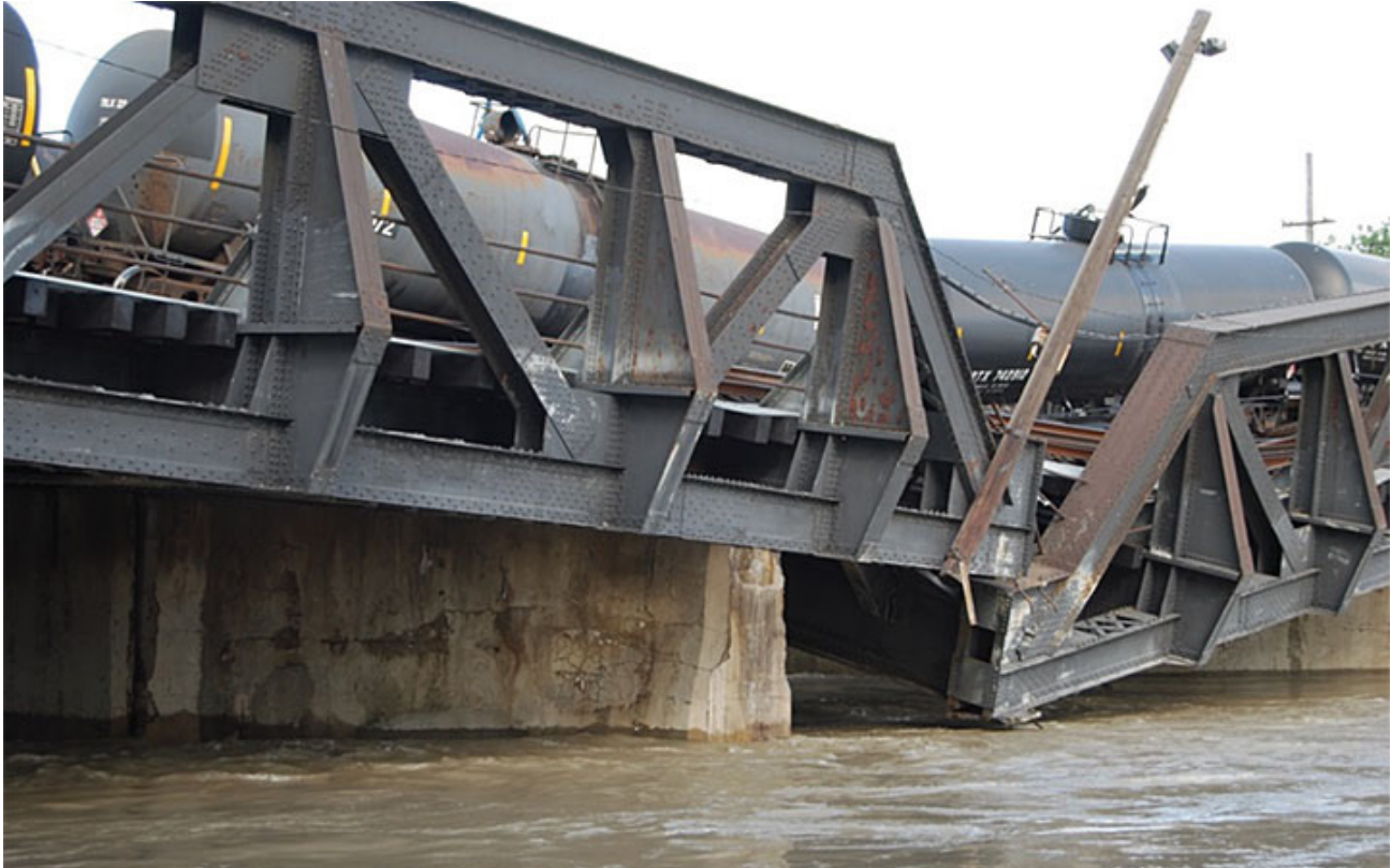
Figure 8: Rail cars sit on the collapsing bridge after a train derailed on Bonnybrook Rail Bridge on June 27, 2013. (Source: Transportation Safety Board of Canada)
