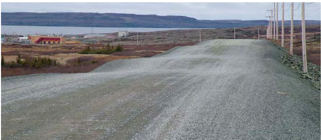
Figure 10: Significant settling on the Umiujaq access road. (Source : Allard, M., Fortier, R., Sarrazin, D. et al., 2007)
