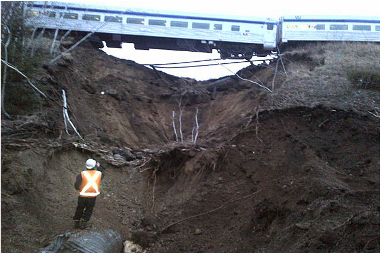
Figure 7: Sub-grade collapse and train derailment due to a frozen culvert in Togo, Saskatchewan, 2013. (Source: Transportation Safety Board of Canada)
