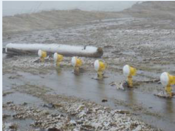
Figure 16: Sandspit runway from December 2011. The end of the runway was subject to severe wave overtopping during a significant storm event, with a sea surge approximately 1 metre above runway elevation. A 250 m section of damaged riprap needed to be re-constructed.
