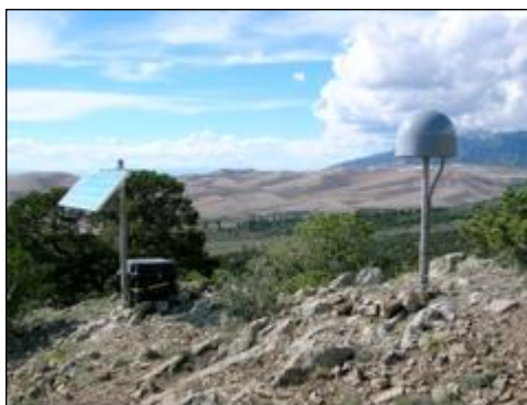
Figure 5 : Braced monument (UNAVCO, 2012)
