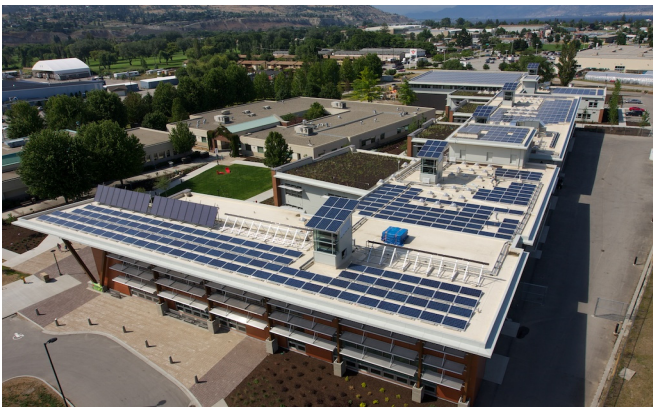
Figure 1: A 260 kilowatt solar PV rooftop system installed at the Okanogan College in British Columbia to meet ambitious target for the living challenge and help train students in green construction practices (Photo: Skyfire Energy)
