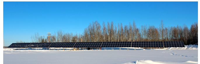
Figure 2: Fort Simpson is Northwest Territories Power Corporation largest diesel-powered community. This 61 kilowatt system (the largest North of 60 degrees in Canada) will help displace 15 000 litres of fuel annually and provide up to 8.5% of the villages' minimum power requirements during the summer. (Photo: Skyfire Energy)
