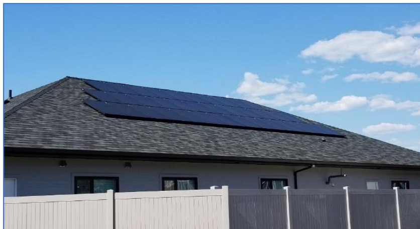
Figure 22: Intended 15 kWp System Limited to 10 kWp by Electric Service Panel Choice - courtesy of Riverside Energy Systems
