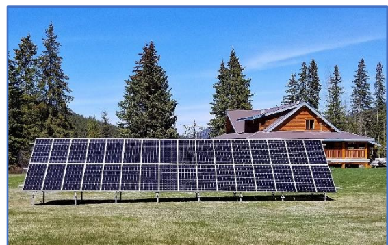
Figure 18: Ground-mounted Solar PV Array - courtesy of Riverside Energy Systems
