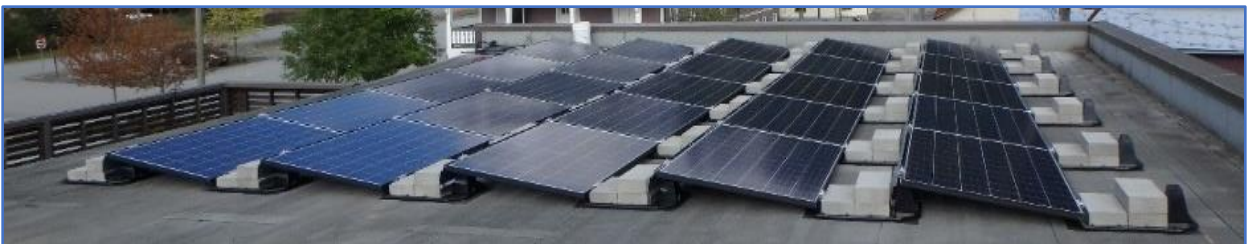
Figure 27: Example of a Flat Roof Ballasted Solar PV Array - courtesy Riverside Energy Systems
