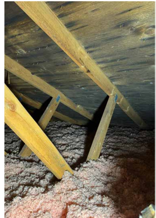
Figure 6 Attic sheathing and framing with visible staining and microbial growth due to moisture accumulation.
