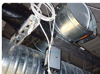
Figure 1 – Zone isolation dampers installed as part of measure 4
