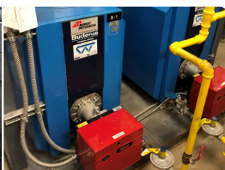
Figure 2 – Boilers that had programming modified as part of measure 5
